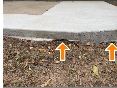
K. Item 2 Soil erosion, back patio
