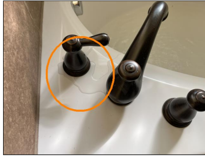
A. Item 4 Master tub, cold water handle
