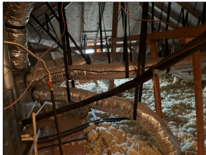
C. Item 1 HVAC duct in attic
