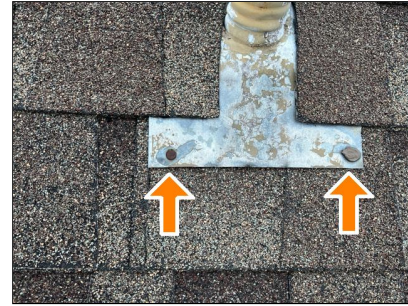
C. Item 5 Exposed nails at flashing
