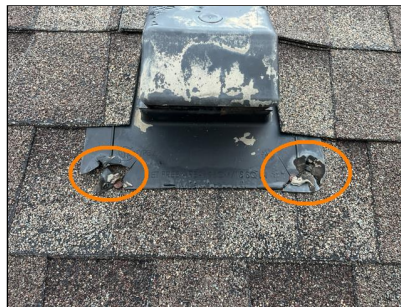
C. Item 3 Dryer exhaust vent flashing
