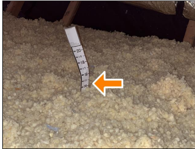
D. Item 4 Loose-fill insulation in attic
