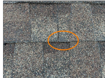
C. Item 8 Wear/delamination
