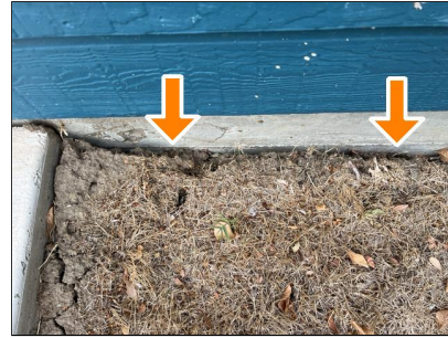
A. Item 4 Foundation, soil separation
