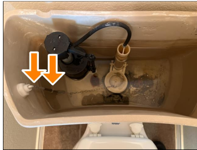
A. Item 5 Handle for flapper valve, master toilet
