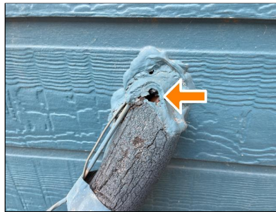
E. Item 4 HVAC line penetration, left side (facing front)
