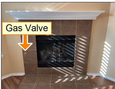
J. Item 1 Gas fireplace
