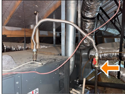
E. Item 2 Gas furnace in attic
