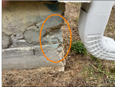
A. Item 8 Corner crack, rear of home
