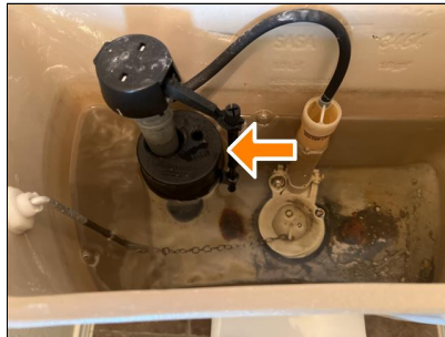
A. Item 6 Float mechanism, master toilet
