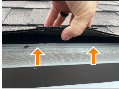
C. Item 1 Improper underlayment on roof
