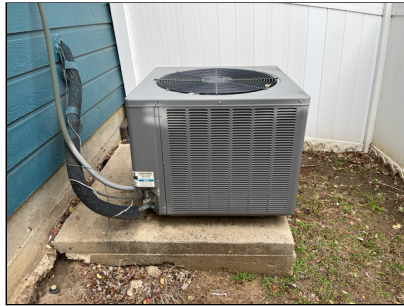
A. Item 1 HVAC condensing unit, left side (facing front)
