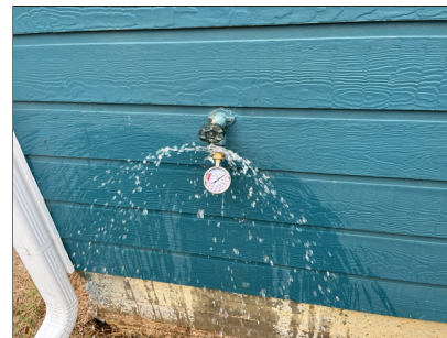
A. Item 2 Hose bib, rear of home
