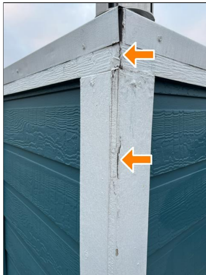
J. Item 5 Wood trim around chimney
