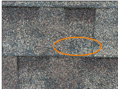
C. Item 7 Wear/delamination
