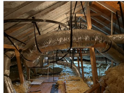
C. Item 2 HVAC duct in attic
