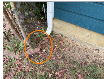
B. Item 2 No splash block and gutter
