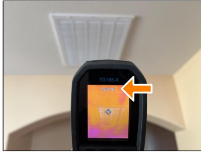
B. Item 4 Temperature reading at air intake on cool setting, 75.7°
