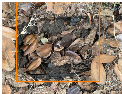
A. Item 3 Water meter, next street
