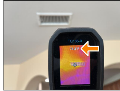
B. Item 5 Temperature reading and air discharge on cool setting, 76.3°
