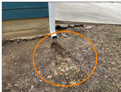
B. Item 1 No splash block and gutter
