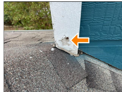
J. Item 6 Wood trim around chimney
