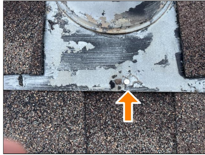
C. Item 4 Exposed nails at flashing
