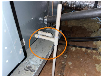
B. Item 1 Condensate drain, HVAC system
