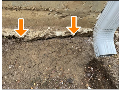
A. Item 3 Foundation, soil separation
