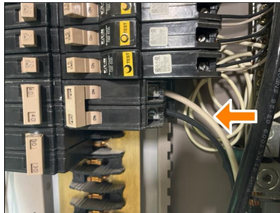
B. Item 2 Improperly-marked wire
