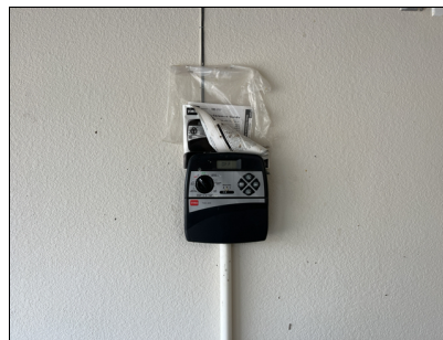
B. Item 1 Sprinkler controller, garage
