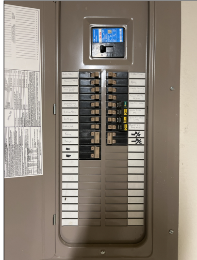
A. Item 2 Electrical service panel, garage
