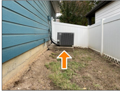
A. Item 3 Concrete pad, condensing unit
