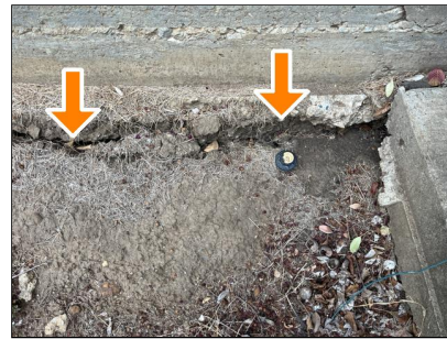
A. Item 6 Foundation, soil separation
